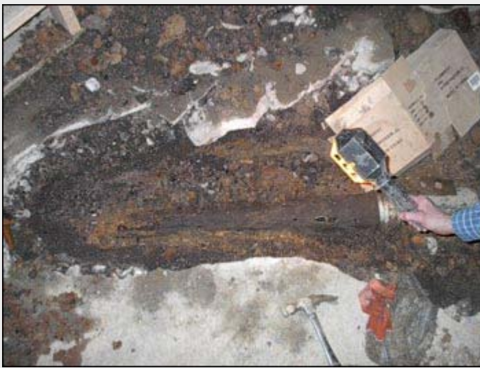
View of corroded sewer pipes under basement slab
